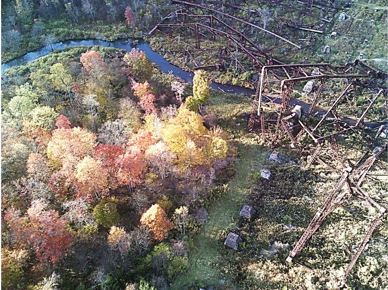
The center part of the trestle was knocked down by massive tornado. The ruins contrast with fall's finest foliage.
